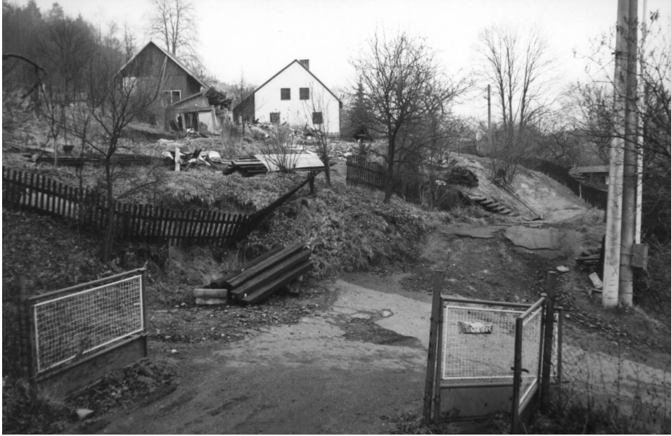
Photo 3: Central part of large landslide with damaged buildings in the Růždka village. (Photo Karel Kirchner)
