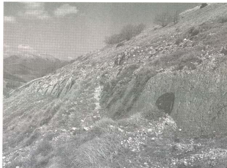
Photo 4 Locality where the Crack Gauge TM 71 was installed on an 8 km long fault trending N-S. The area did not show any signs of slope movements which could affect the monitoring (Photo by V. Vilimek)
