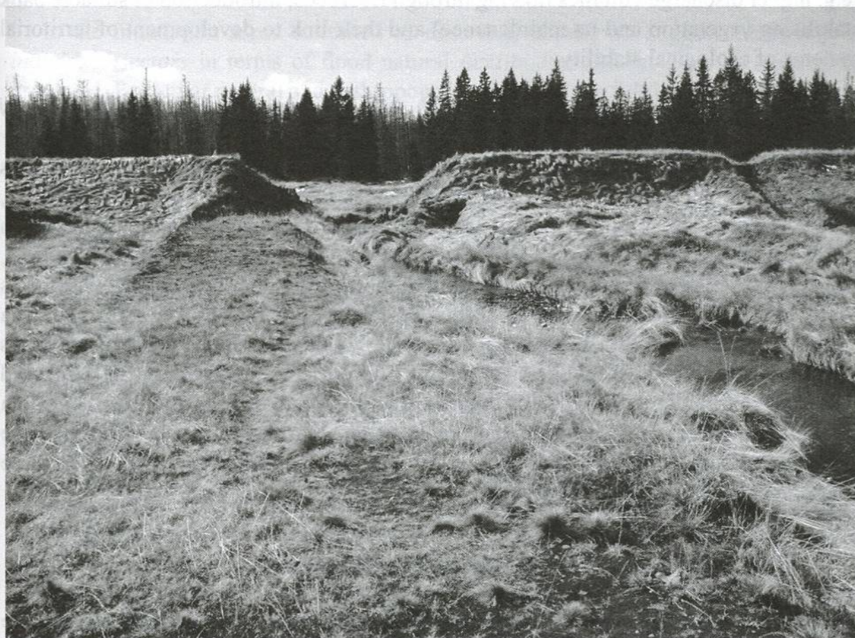
Fig. 2 Broken dike by Roklan forester's house (Photo T. Hrdinka)
