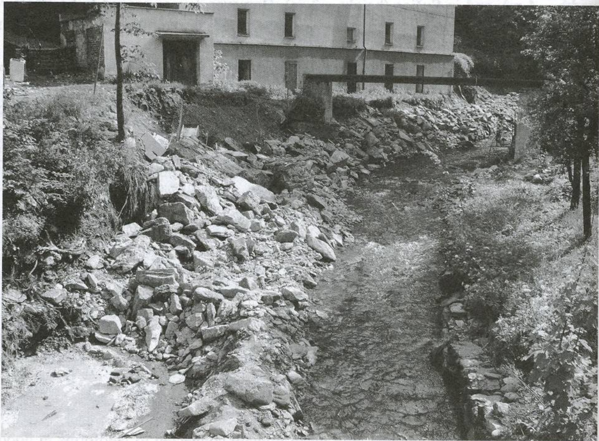
Photo 4 Damaged flood-control levees and anthropogenic reinforced bank in the Volyňka river in Vimperk. It is a result of anthropogenic restriction of the river bed capacity (Photo by M. Křížek, 2003)
