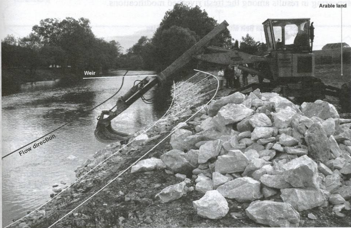
Fig. 4 Reconstruction of river bank pavement damaged by the flood. The river segments located under the weirs were frequently points of intensive erosion and accumulation as result of the flood in August 2002 (Photo J. Langhammer, 2003)
