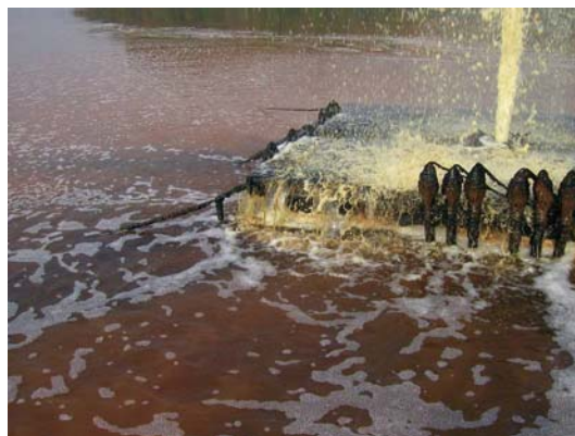
Fig. 9. Ferric oxyhydroxide build-up on control valves. 800 kg of precipitate had to be removed from the Nyos raft to prevent sinking.
