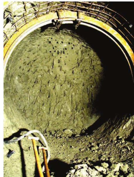
Figure 3. Circular adit used in backanalyses of the earth pressure coefficient at rest K_0 (Pavlik et al., 2004).
