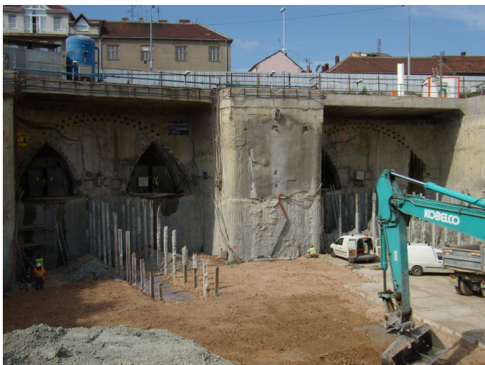
Figure 3. Exploratory drifts situated in the top headings of the future Královo Pole tunnels.
